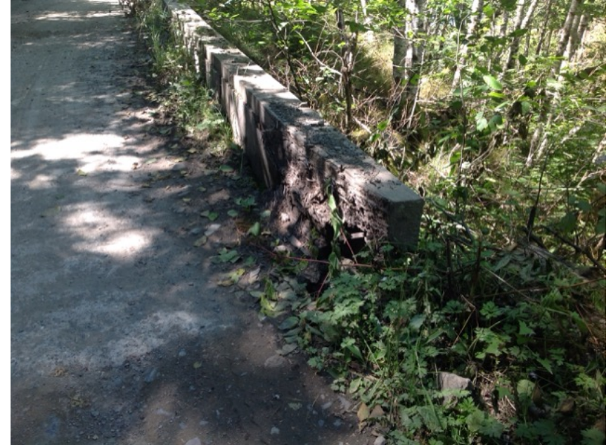
damage to downstream guardrail but still functional
